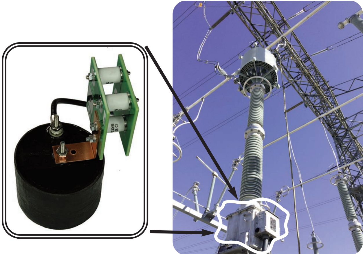
Close Up of Smart Gap Mounted on the Drain Coil (Left) and Location Inside Coupling Capacitor / CCVT Base Housing (Right).
