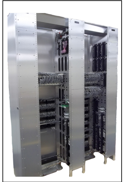
Rear view of Lucasey Rack with TR-3000, ABB FT-19R test switches and GE EB-25 terminal blocks.
