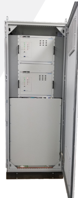
Rittal Cabinet with TR-2200.
